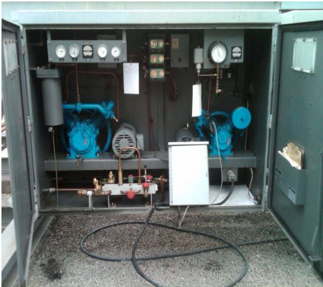
Fig. 7. The CBR device next to the open CB cabinet
