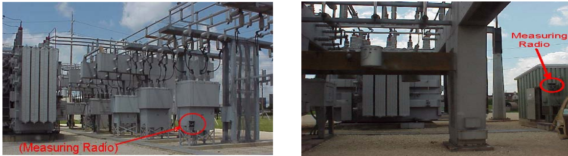
Fig. 3. None-line-of-sight (NLOS) disposition of the instruments in a power substation
