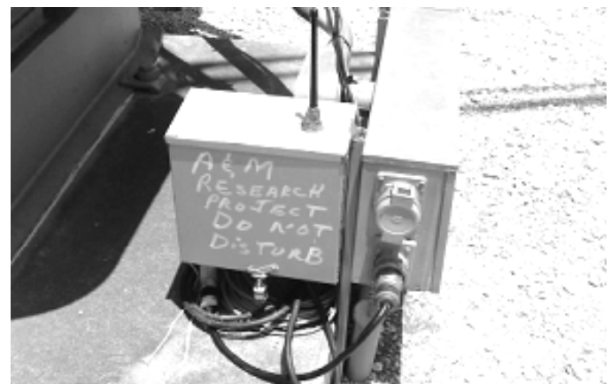
Figure 9: CBM device installed in switchyard
